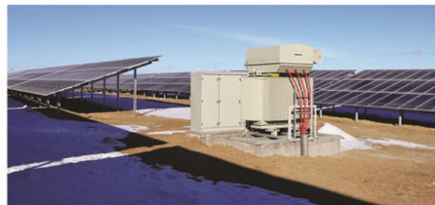
Hamedan Solar Power Plant
